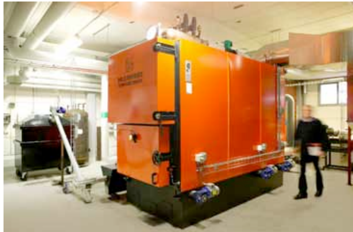
Biomass boiler with NovaReg control both from ABioNova
